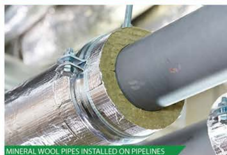
MINERAL WOOL PIPES INSTALLED ON PIPELINES
