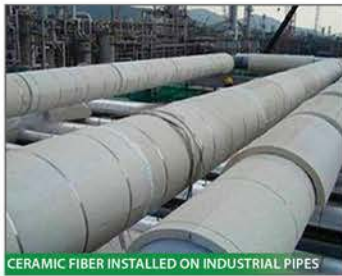
CERAMIC FIBER INSTALLED ON INDUSTRIAL PIPES
